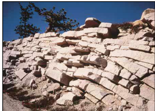
Figure 2–3 Pressure-release fracturing contributed to the formation of these cracks in a granite cliff in Tuolumne Meadows, California.
