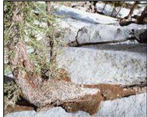
Figure 2–6 As this tree grew from a crack in bedrock, its roots forced the crack to widen.
